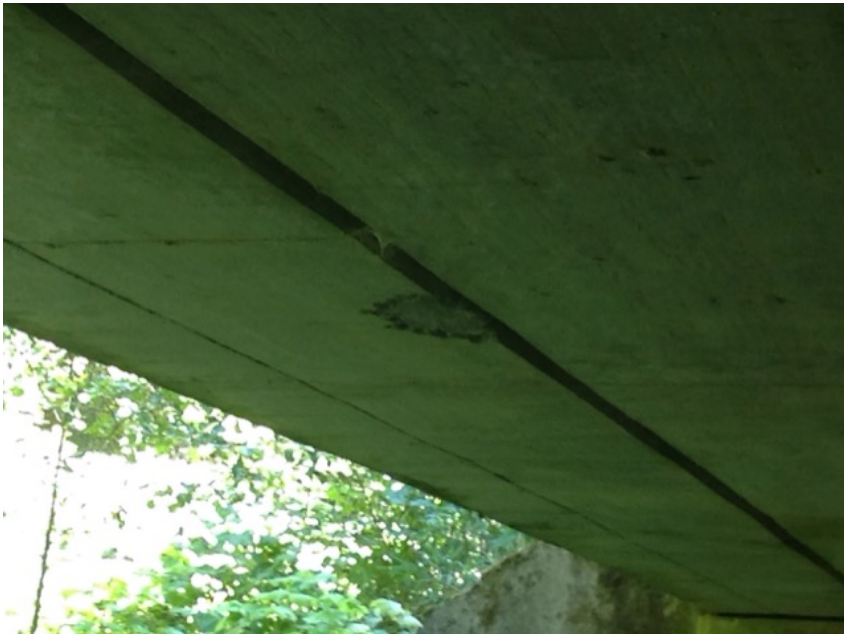
spall that was grouted
