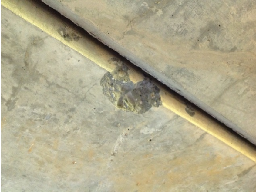
minor spalling on left bank 6th slab
